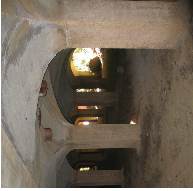
Structurally unsafe groin vaults and columns
